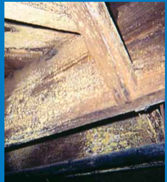
Mold clings to floor joists, degrading the home's structural integrity.
